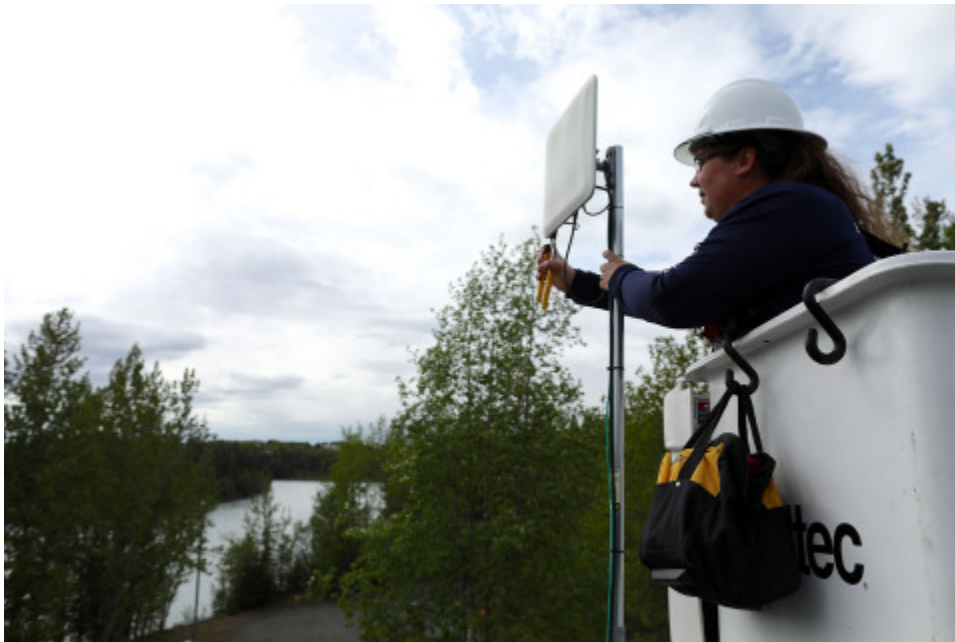
Alaska Communications Field Technician Kristine Barber installs fixed wireless at a home in Sterling, Alaska. (Photo: Business Wire)
